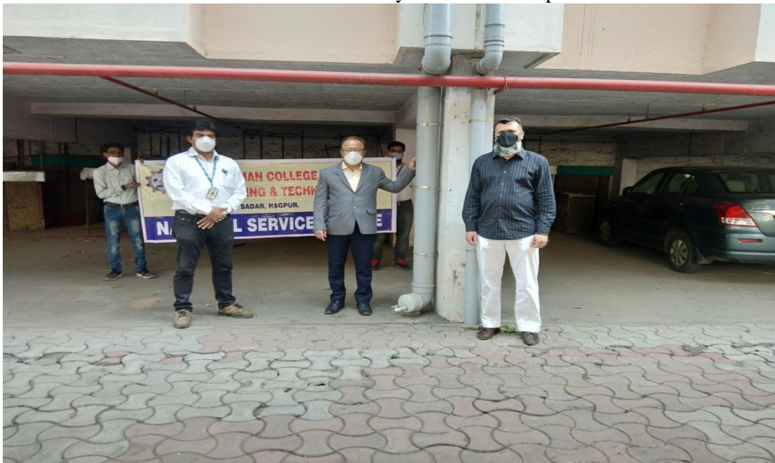
1) RAIN WATER HARVASTING PIPES (Pipes from roof top)[Ground floor Vehicle Parking Area]
