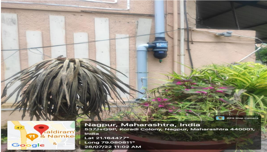
2) RAIN WATER HARVESTING PIPES WITH FILTER ATTACHED(Pipes from Roof Top of First year building)
